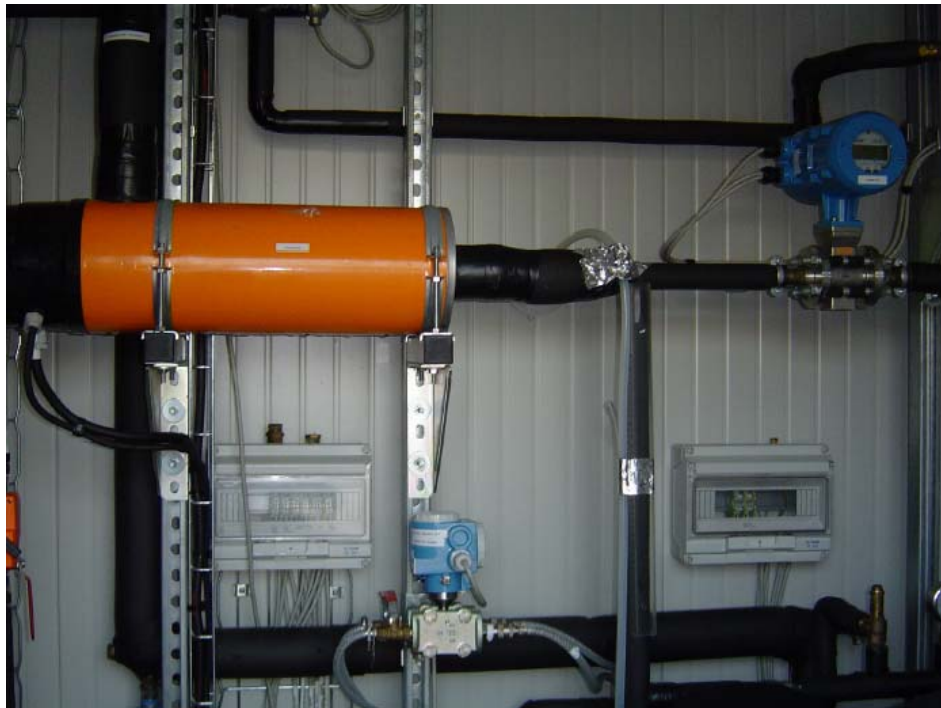
Figure 4. The electric heater.
